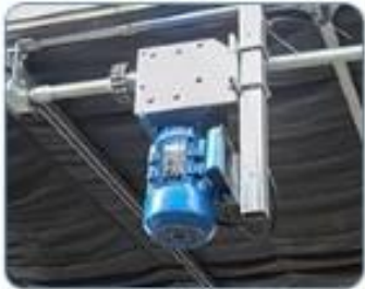
Automatical Curtain System
